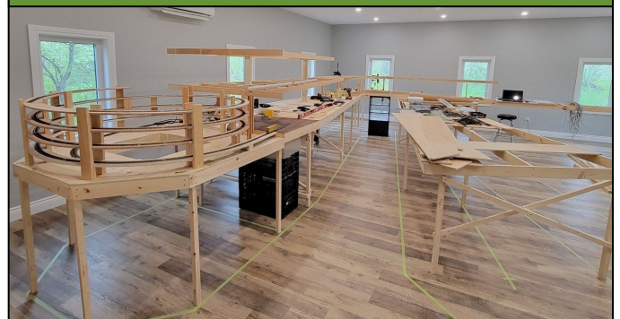
Photo Below: May 8, 2024: This photo taken, shows the helix construction and the beginnings of the center peninsula.
